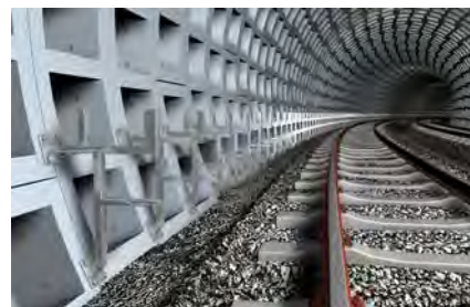
Instalace v tunelech
